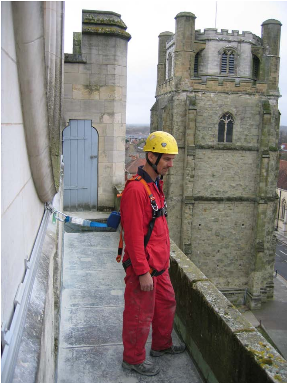
Unirail lifeline fitted to the North Nave Transept gable end, Chichester Cathedral.
