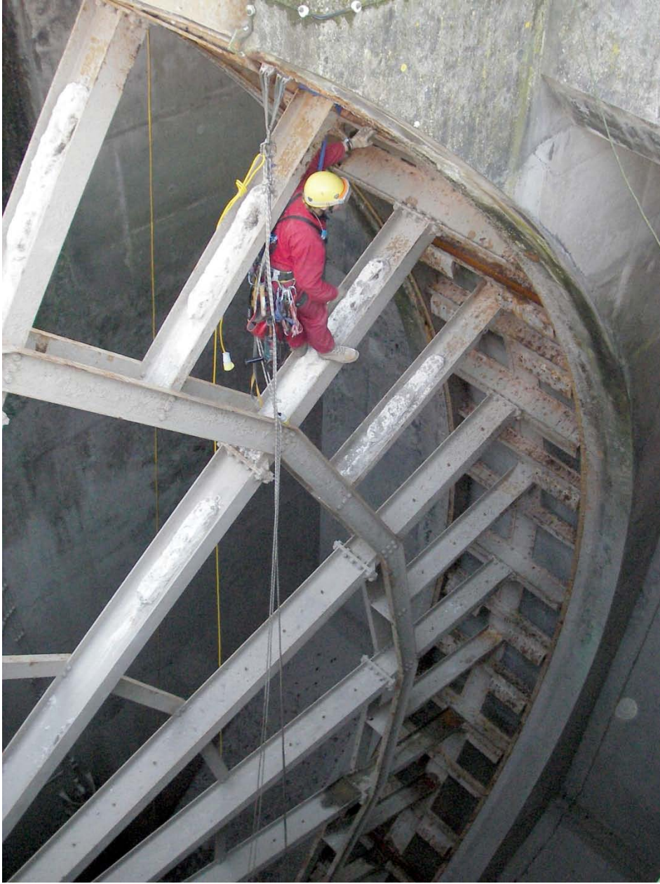
Inspecting the lift buckets for damage.
