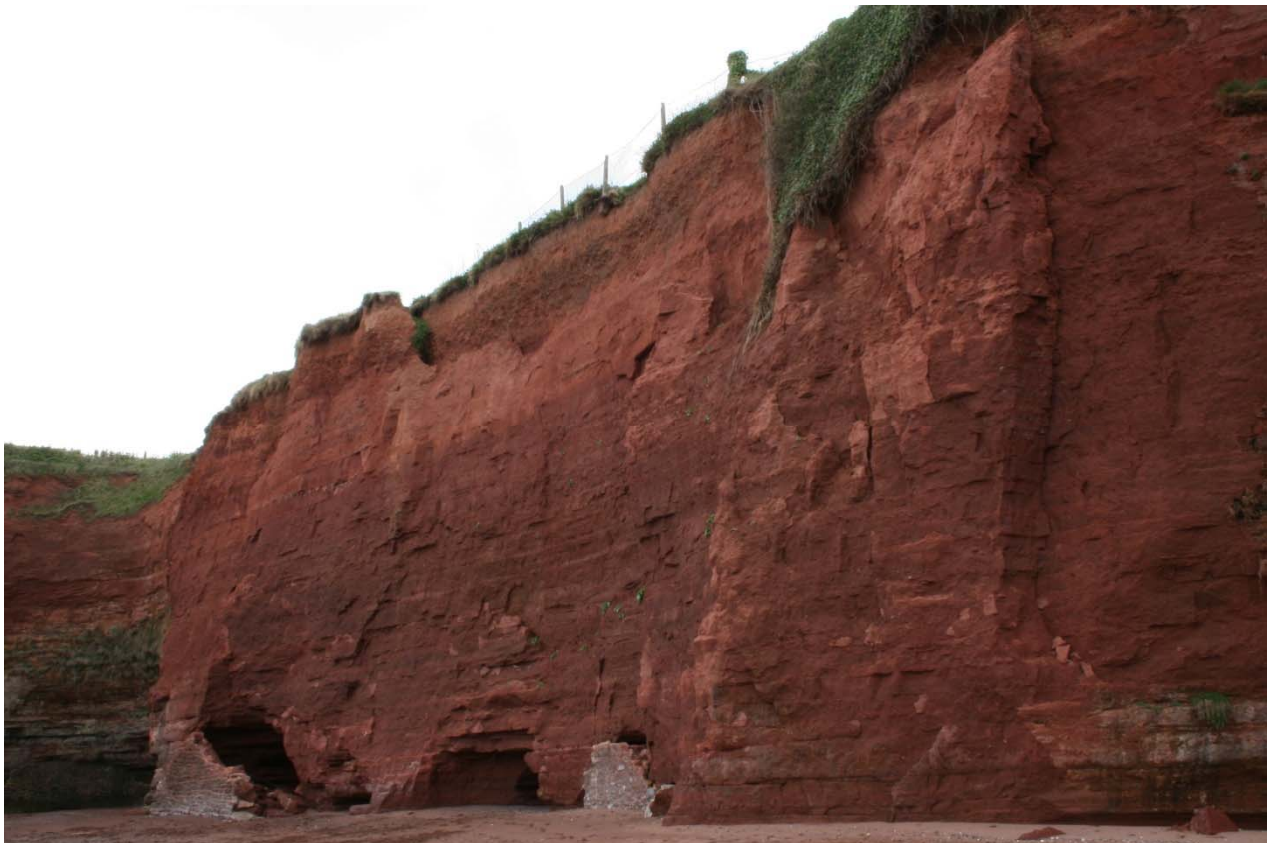
Hollicombe bay cliffs prior to remedial works
