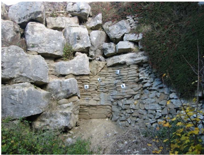
Other areas required temporary propping to allow safe access, dentition and hollow anchors
