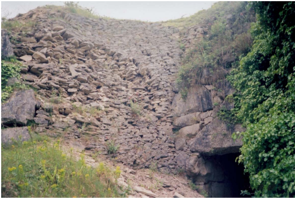
A typical section of collapsing dry stone retaining wall
