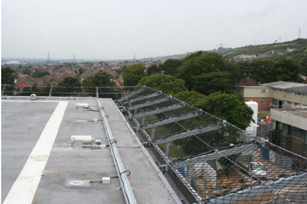
With no edge protection and the spars in an awkward location, roped access was widely used to install the heli-pad safety fence.
