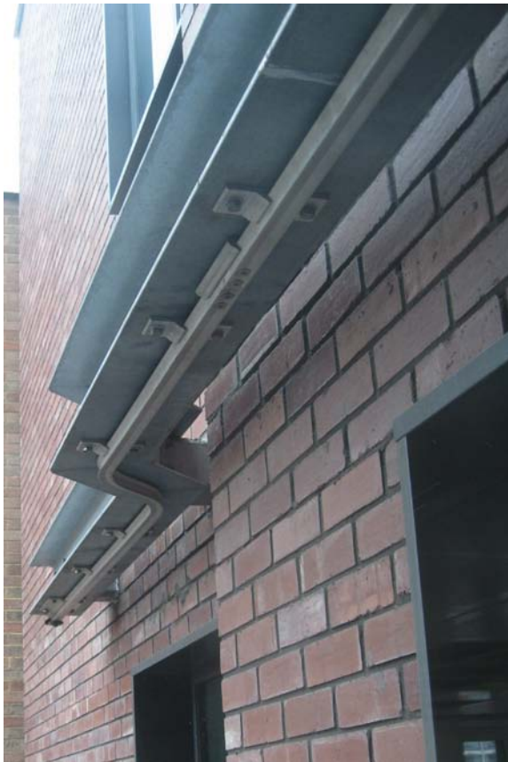
Unirail abseil rail system fitted to steelwork running around a lightwell.
