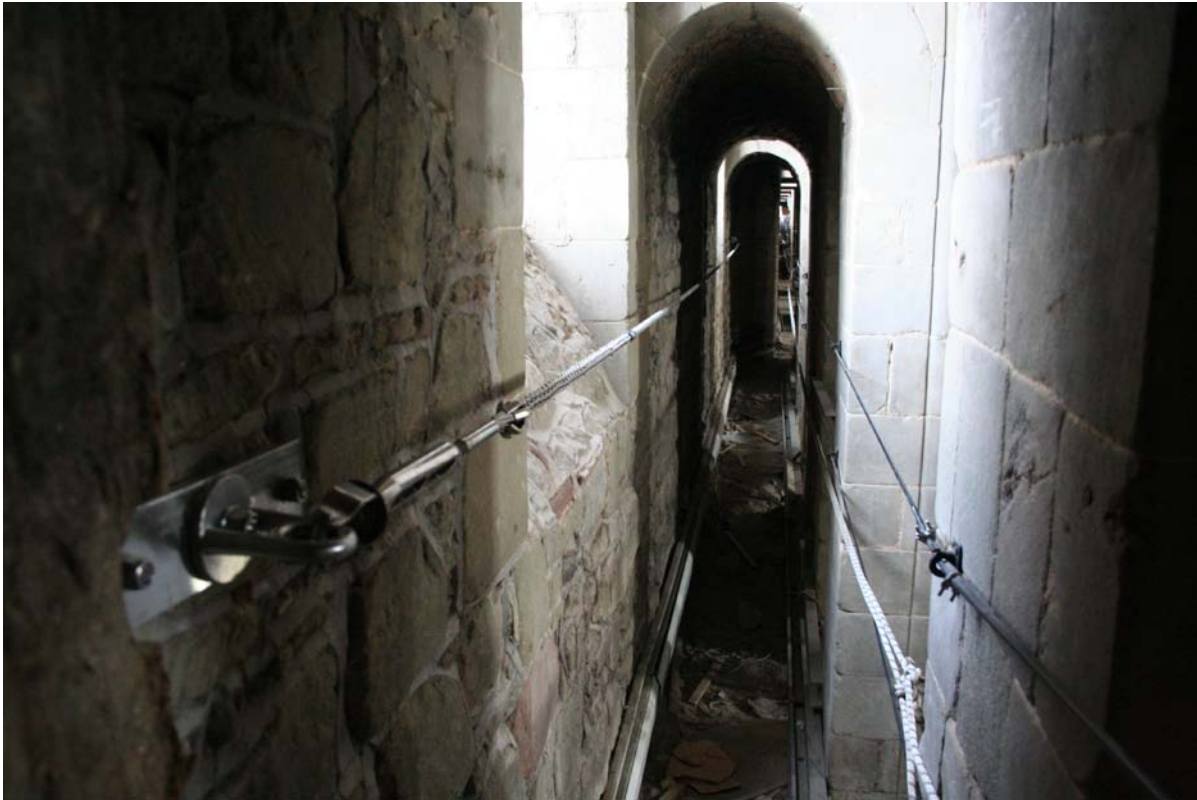
Uni16 lifeline running the length of the high level clerestory.
